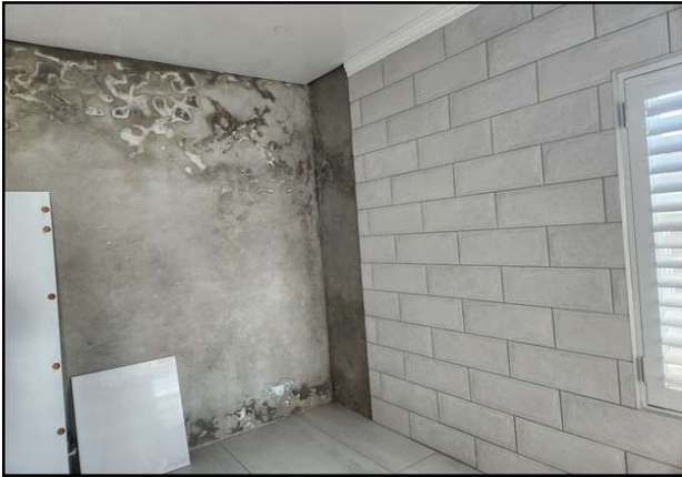
Incomplete dressing room:
